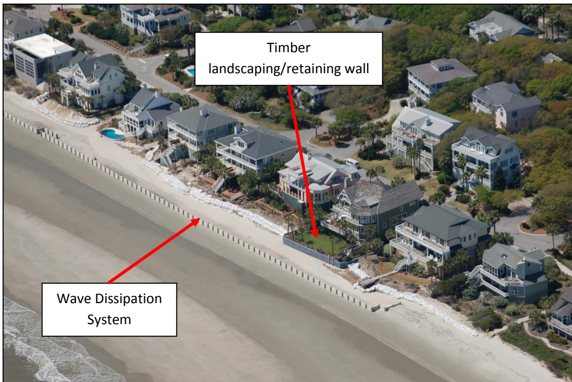
Figure 20. April 5, 2016 photo of Wave Dissipation System installation at Beachwood East (same area as shown in Figure 16). WDS ties into rock revetment at west end, see Figure 19. A timber retaining/landscaping wall is also shown. The Wave Dissipation System was removed in 2018.
